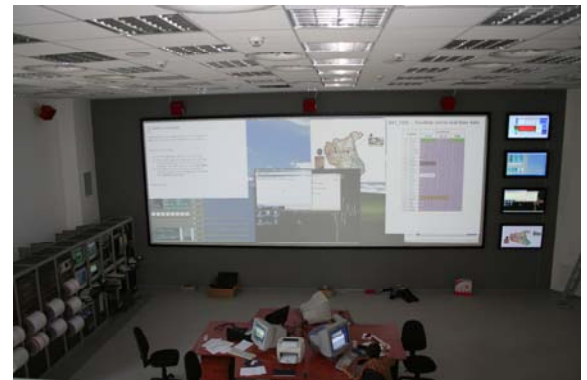
Romanian National Data Centre
